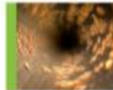
▶ PITTING Min. 10% of wall thickness
